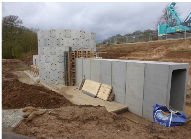
North site control structure
